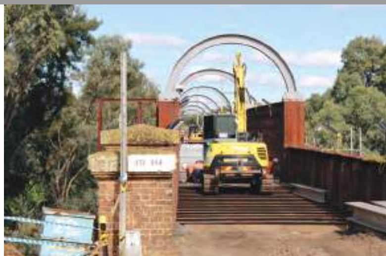
Installation of over 300 galvanized cross-braces required a round-the-clock effort to ensure this vital bridge link was returned to operation on schedule.
