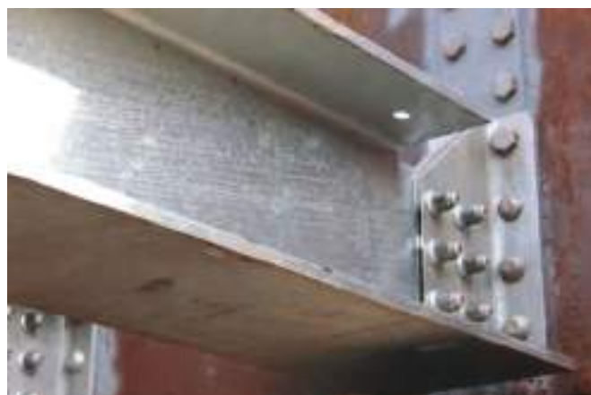
Riveted fasteners were replaced to facilitate speedy removal of the old cross-beams during the 16-day outage.
